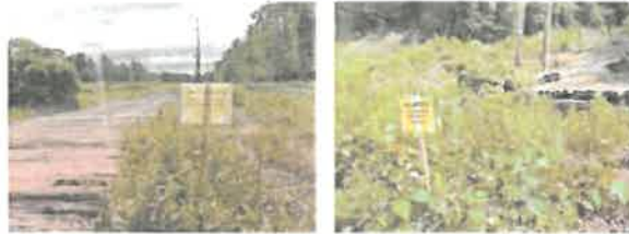
NO ACCESS – WETLAND/STREAM CROSSING MATS REQUIRED
