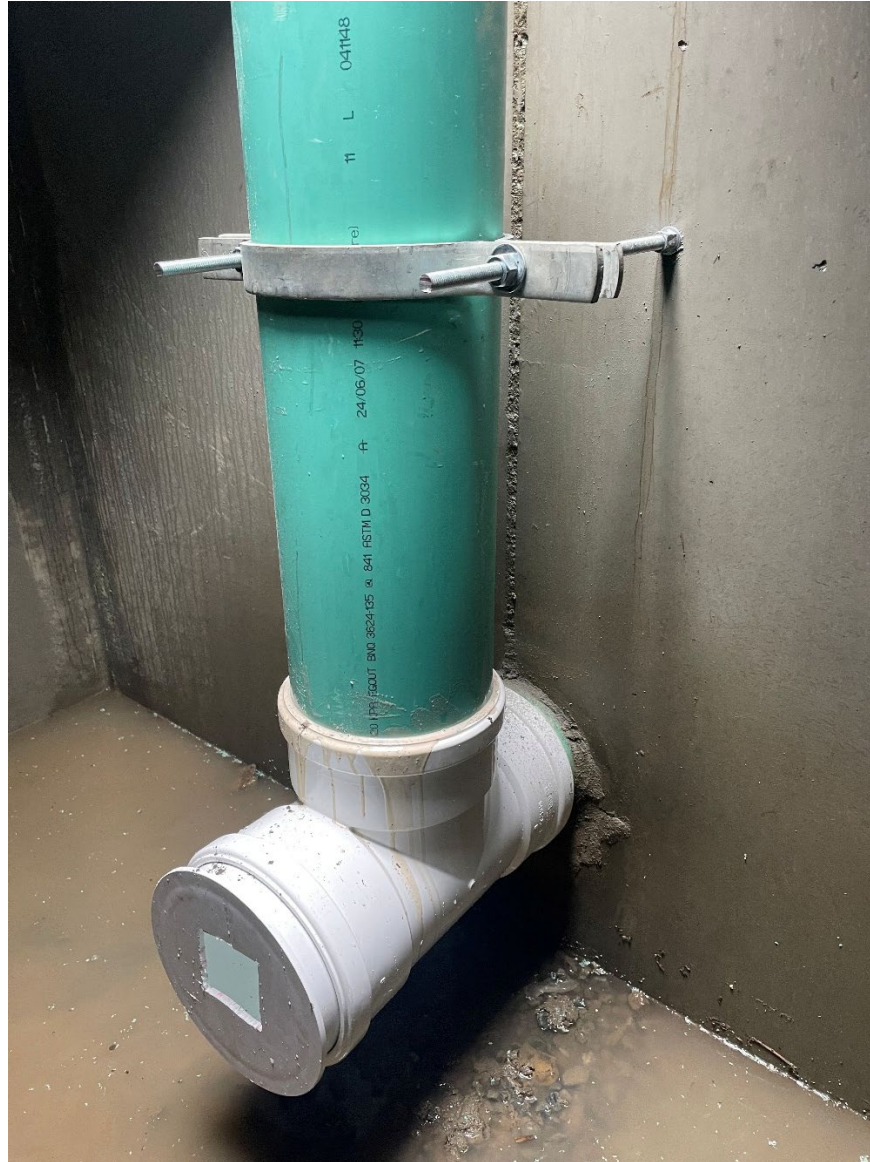
Comment 17.A response backup (Outlet Control Device)
