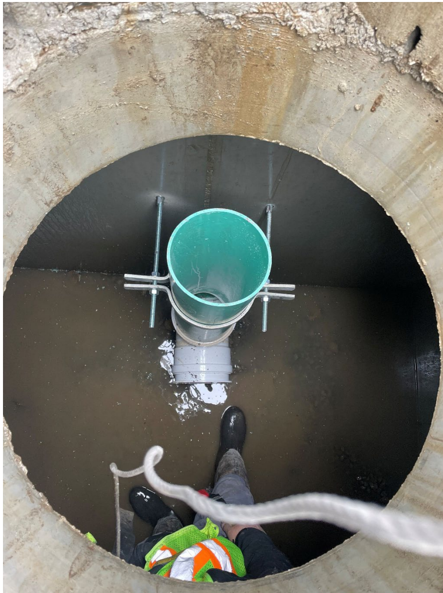
Comment 17.A response backup (Outlet Control Device)
