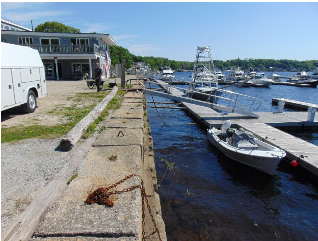
Photo 8 – View northeasterly along retaining wall along the edge of the Merrimack River where a few portions of the retaining wall were observed to be loose. The existing marina building is at the upper left of the photo.
