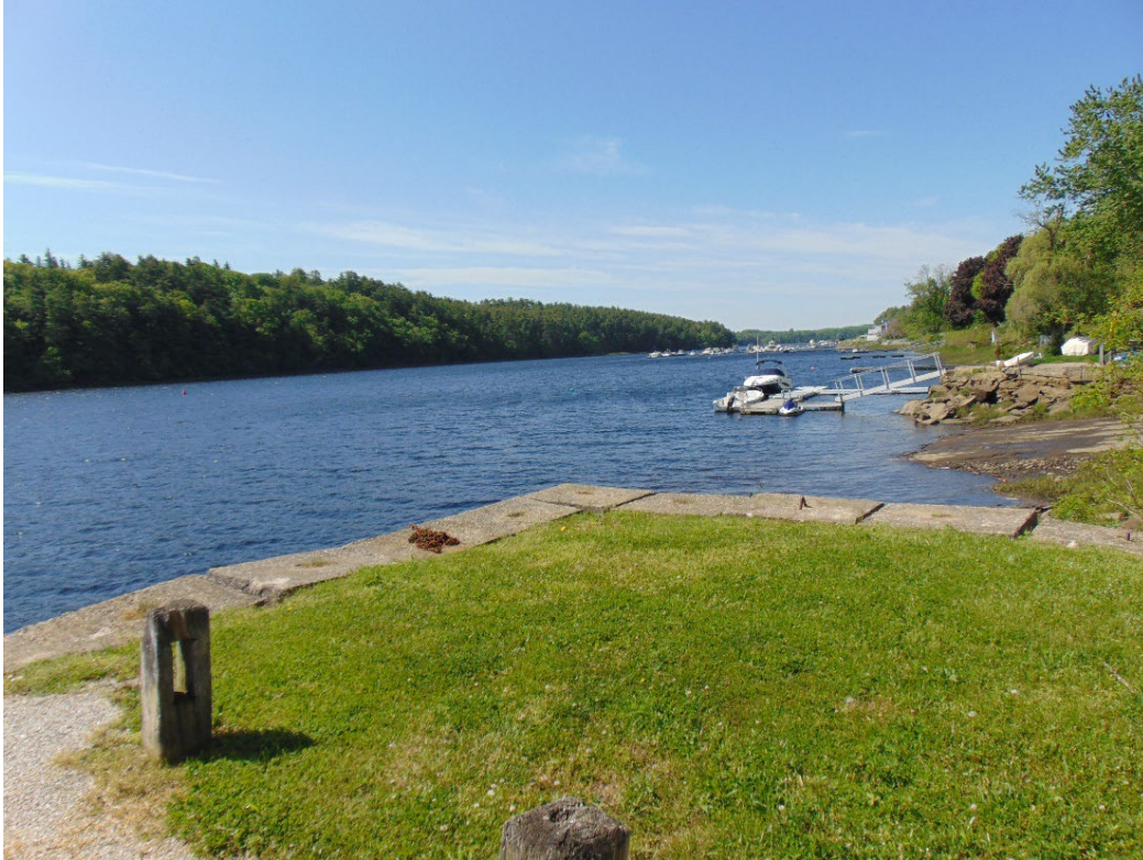
Photo 7 – View southwesterly along the westerly property line near the property corner at the Merrimack River where a few portions of the retaining wall were observed to be loose.
