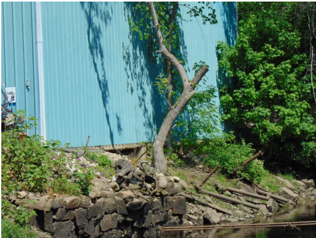
Photo 10 – View northwesterly along the Pow Wow River and of the existing foundation of the building to remain in need of repair. Some invasive species appeared to be present along the embankment.
