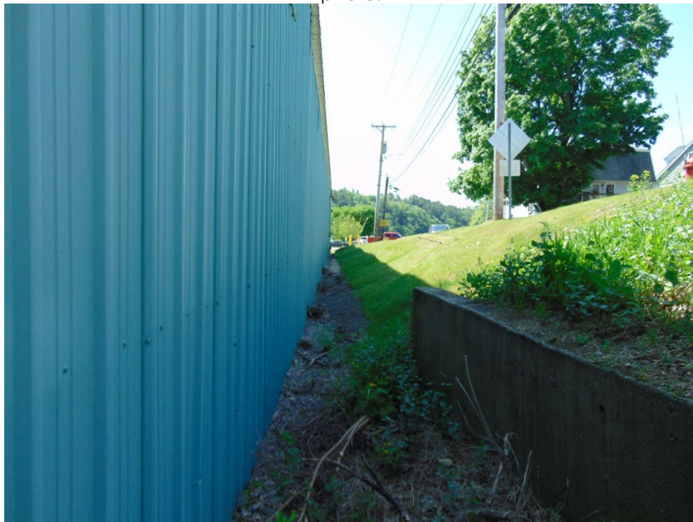
Photo 6 – View southerly from the northwesterly corner of the site adjacent to the westerly side of the building looking along the Merrimac Street roadway embankment. A proposed retaining wall would impact the existing roadway embankment. The existing retaining wall is seen in the lower portion of the photo.
