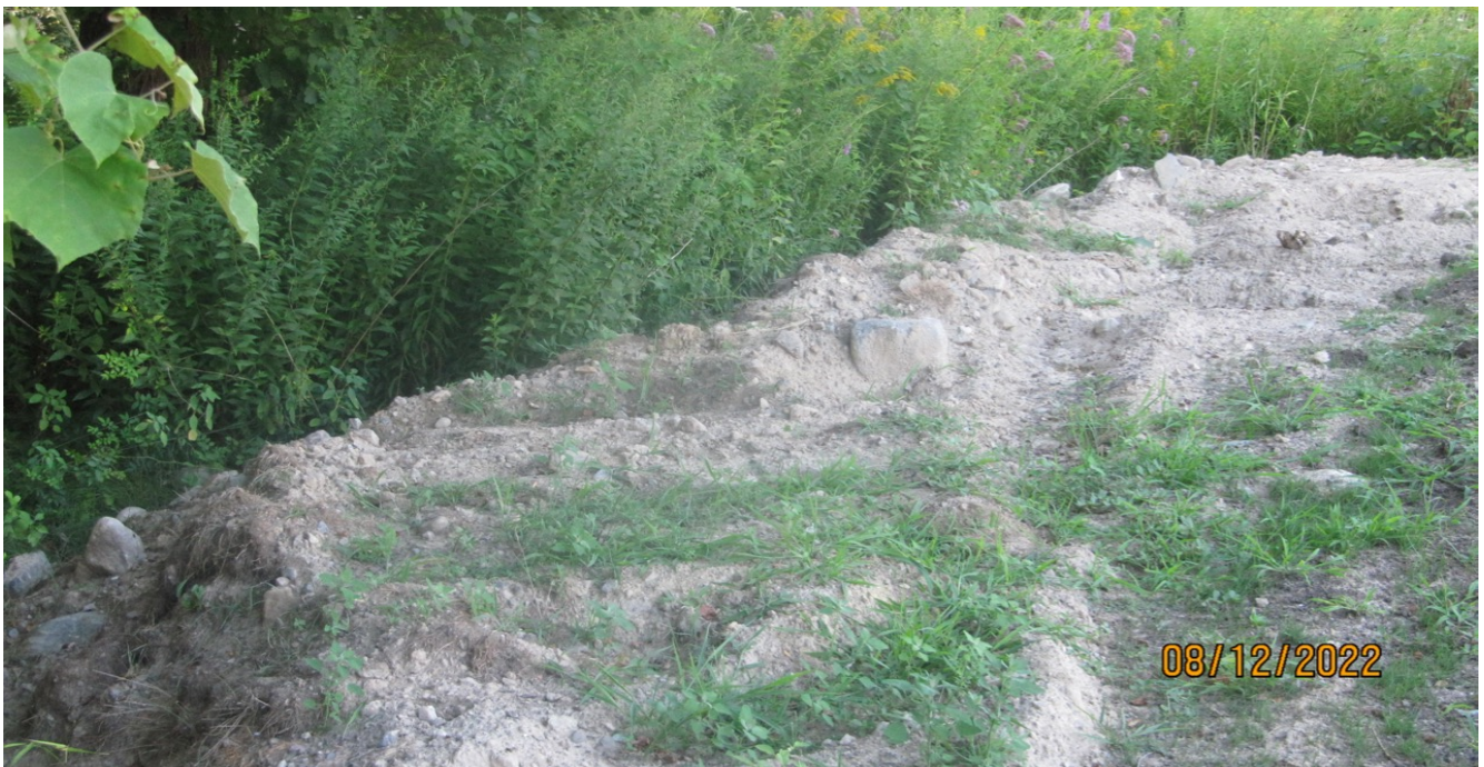
Photo F. Edge of fill still not regraded at northwestern edge of fill area. No coir logs were installed in this area as recommended.
