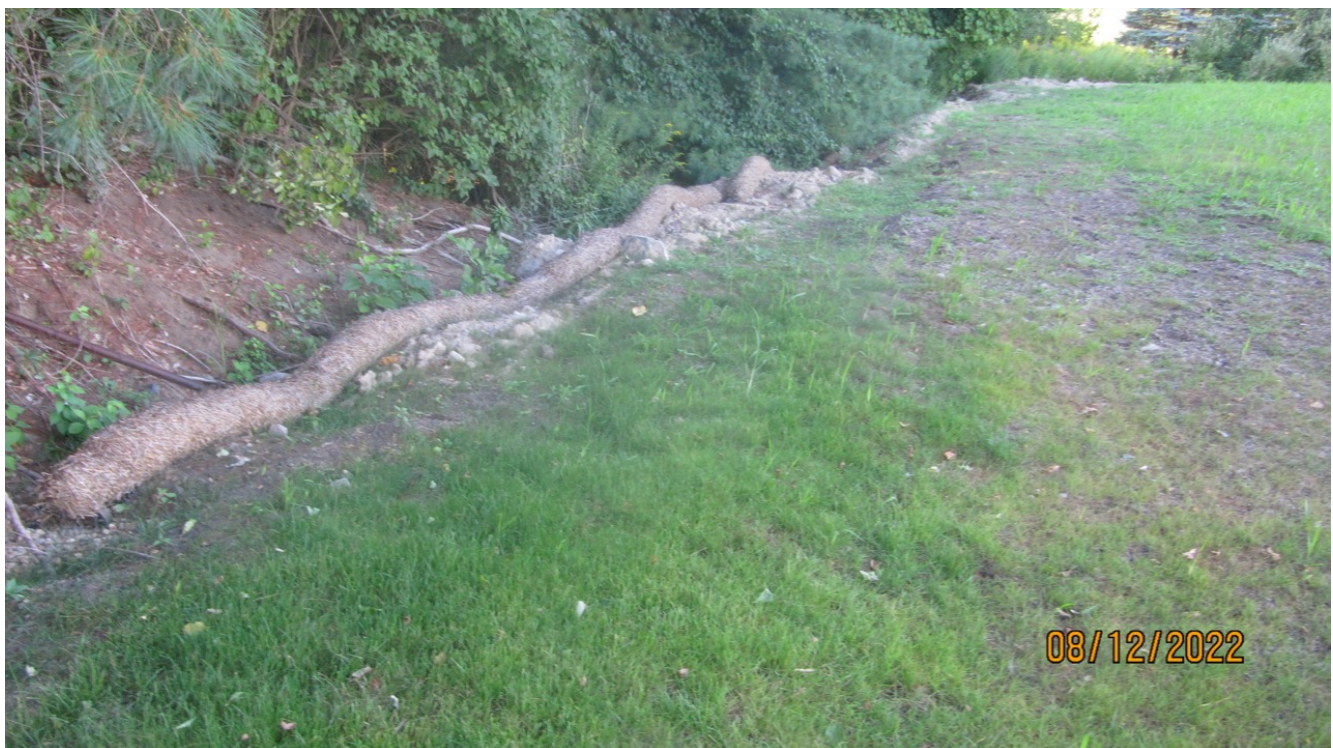
Photo D. Coir logs still in place, but stakes in the logs were not been installed as previously recommended.
