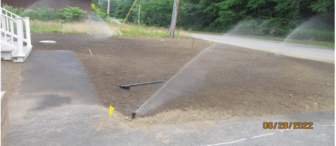
Photo G. A portion of the new sprinkler system installed in the front yard.
