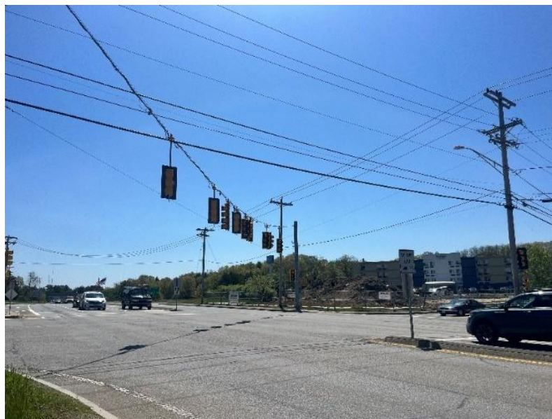
Figure 9: Macy Street (Route 110) at Elm Street and Clark's Road faded markings
