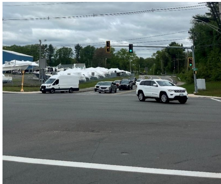
Figure 13: Signal heads on the north leg of the intersection, two with retroreflective backplates and one without
